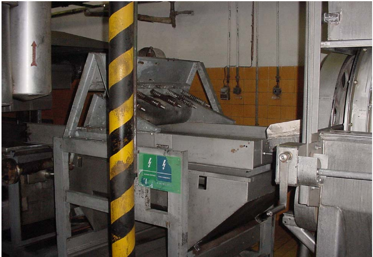
Pos 5 Dewatering Fryer Infeed Vibrator
